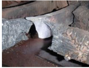
10. Arc damage was found at the joint between the stator bar and connection ring
