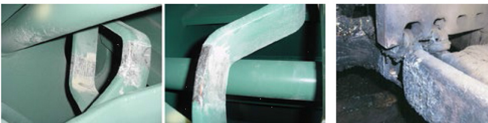
6, 7. Insulation wear on two rings in different phases is clearly problematic 8. Arc damage was caused by failure of connection-ring insulation
