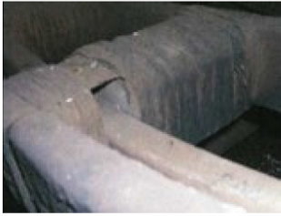
9. Questionable blocking of connection rings was in evidence on a winding that failed in service
