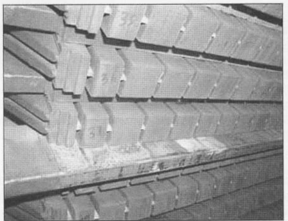
Figure 7 Bar abrasion due to loose windings in the slot of a turbo generator that did not have sufficient sidepacking or a radial follow-up wedging system.
