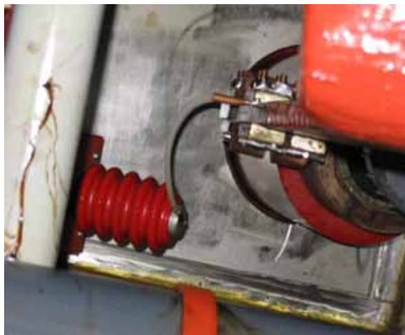
Fig. 1. 80 pF capacitive coupler inside housing of 300 MVA machine
