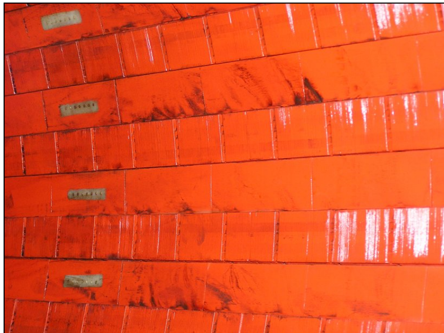
Figure 2-6 “Greasing” Seen at the Slot Wedges
