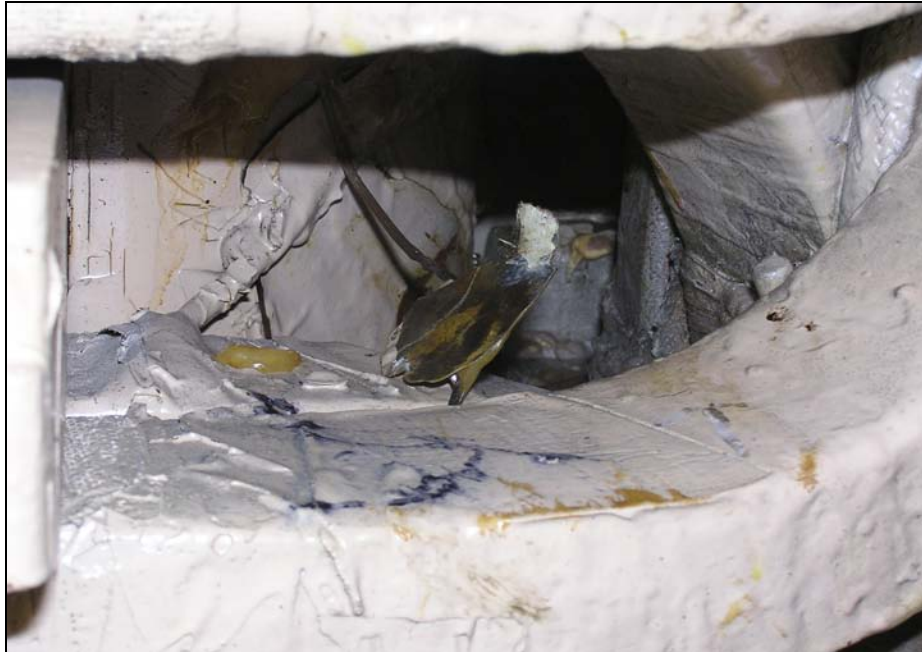
Figure 3-13 Debonded and Severed Flux Probe Wiring (See Text)
