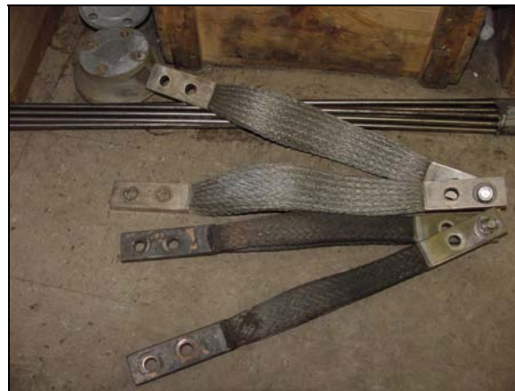
Figure 4-15 Two Levels of Overheating Previously Observed on Leads from Marshall #3
