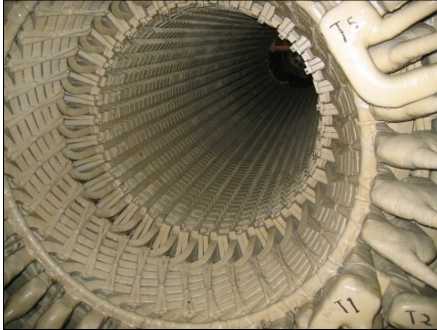
Figure 4-11 Overall View of the End-Winding Region of Marshall Unit #4
