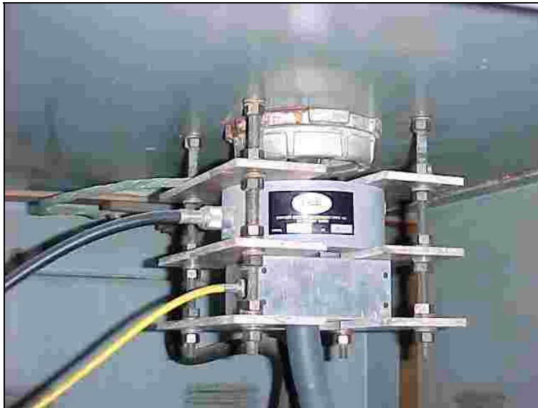
Figure 2-5 High-Frequency Current -Transformer at the Machine Neutral
