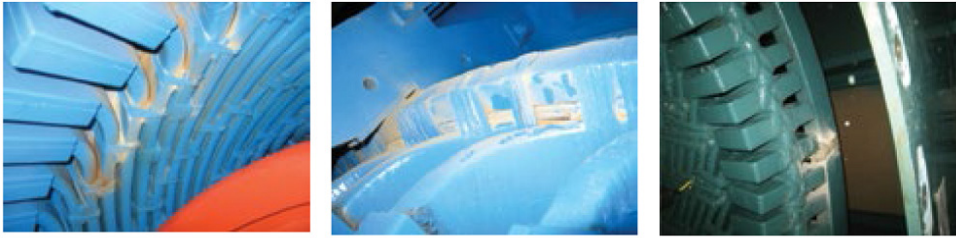
1, 2, 3. Dusting is indicative of early-stage vibration in endwinding
