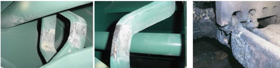
6, 7. Insulation wear on two rings in different phases is clearly problematic
