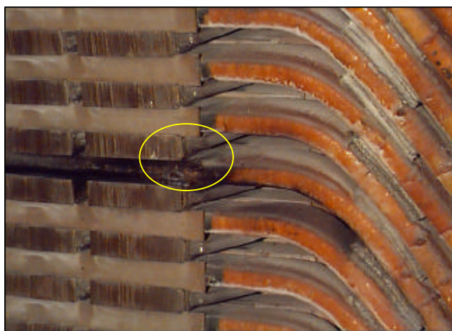
Fig. 4 Visual inspection of the insulation failure.
