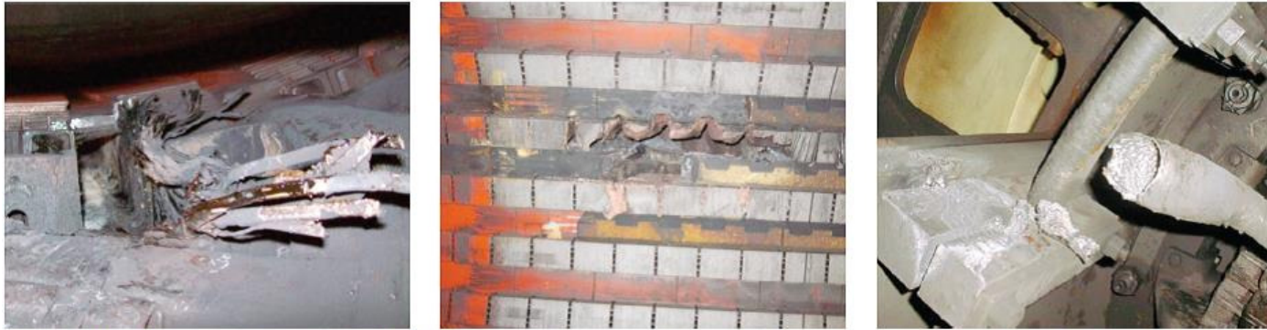
7-9. Failure-to-ground caused by the fracture of a stator conductor is not rare; examples are shown in these three photos. Core and winding damage attributed to a burned open bar in a slot is shown in the left and center photos and the burned-away copper of a fractured connection is at the right
