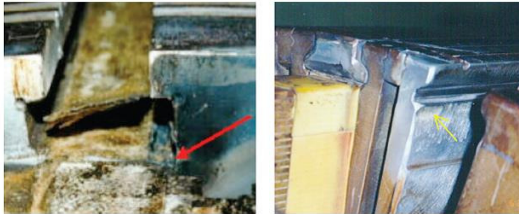
1, 2. Minor rotor-forging burn damage (left) in an area of low mechanical stress is relatively easy to correct by light grinding of field iron, as shown at the right
