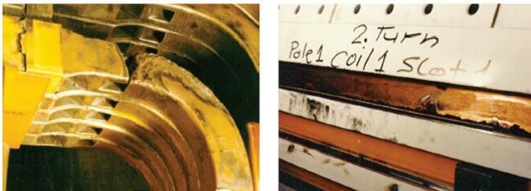
3, 4. Single-ground failure initiated by a broken top turn (left) caused serious burning of the forging and copper (right) when current continued to flow
