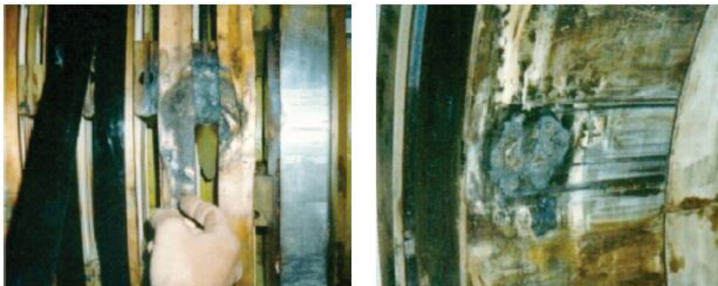
5, 6. Arc damage from shorting between two coils (left) effectively removed the coils from the excitation circuit. The single ground lasted for a significant period of time because the detection circuit was connected incorrectly. Result: Near-fatal burn damage to the retaining ring (inside diameter)
