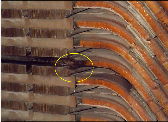
Fig. 3 Location of the insulation failure.
