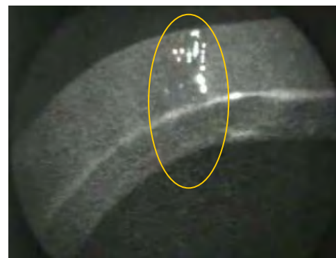
Figure 6 – UV camera view of the corona discharge at the junction – Case 1
