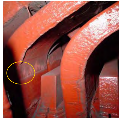
Figure 1 – Signs of discharges on a winding after just four years of service
