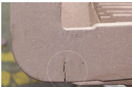
9. Tired turn. Low-cycle stresses can lead to fatigue cracking of copper turns. The resulting arcing and burning can cause short-circuits and rotor imbalance. Courtesy: National Electric Coil
