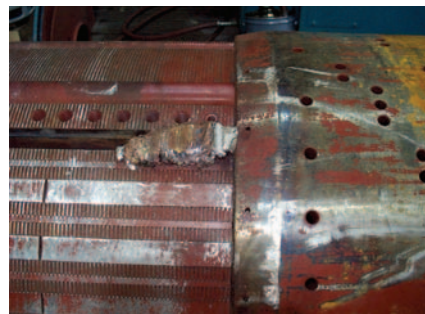
8. Wreaking havoc. The failure of a rotor slot wedge also can produce severe damage. Courtesy: National Electric Coil
