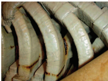
4. Vibration's damage. The greasing between the coils is symptomatic of end-turn vibration. The grease results from the mixing of entrained oil with particles of insulation dislodged by the relative motion of coils. Courtesy: National Electric Coil
