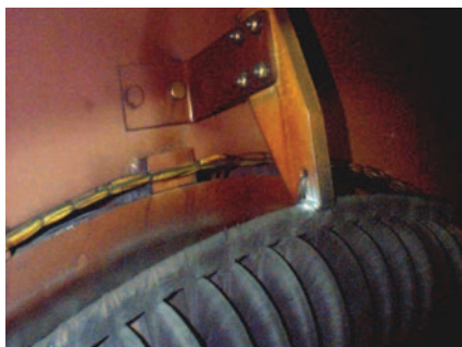
5. Ah, there's the rub. Note the white powder where the bracket and the end turn surge ring meet. The dusting was created by the relative movement of the stator coil's end turns and the support bracket. Courtesy: National Electric Coil
