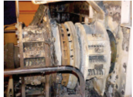
19. Catastrophic failure was caused by a flashover between polarities
