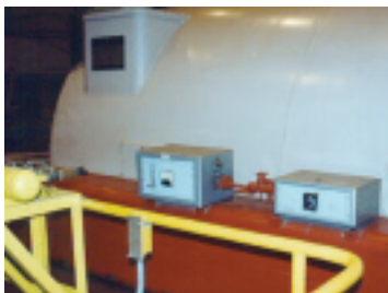
3. Condition monitor identifies any source of excess temperature
