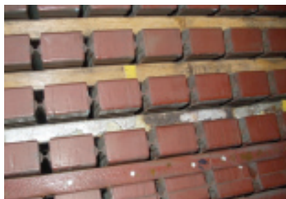
7. Advanced partial discharge activity is in evidence on bar surface
