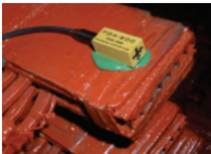
1. Stator end-winding vibration sensor is mounted on a winding series connection
