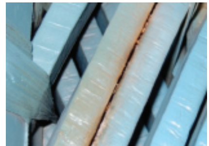
11. Partial discharge attack is in evidence at line-to-line phase break
