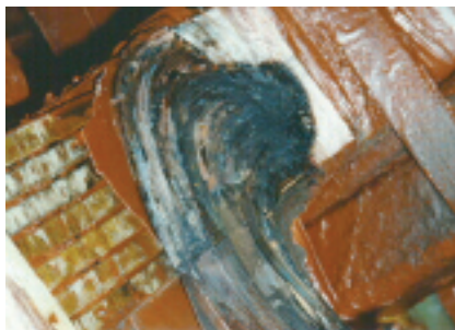
9. Failing series connection was identified on stator end windings
