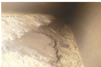
8. Spark damage caused by vibration is seen in ventilation duct through a borescope
