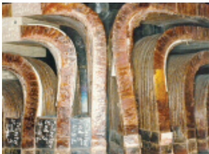
16. Significant coil/turn distortion is evident with the retaining rings removed
