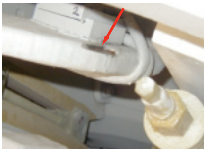
10. Foreign-object wear has left bare copper exposed
