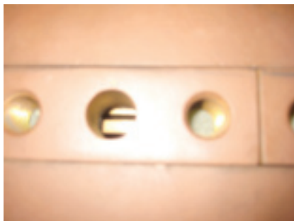
17. Inspection via ventilation holes in the wedges is possible on direct ventilated fields
