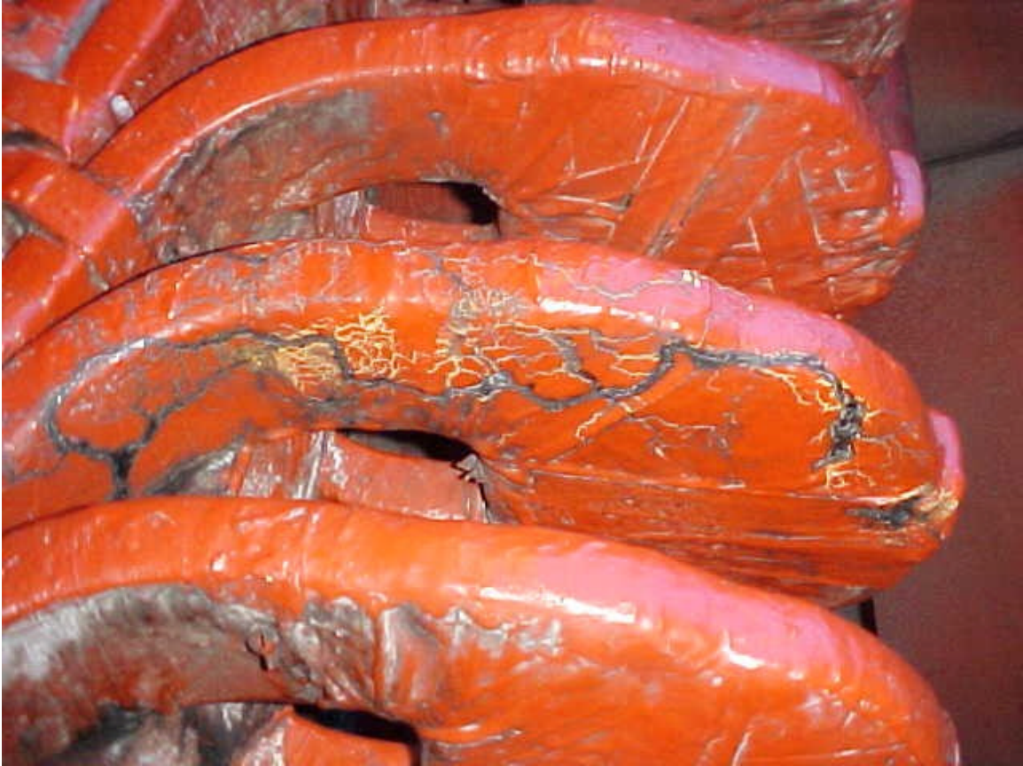
Figure 3: Photo of phase to ground electrical tracing over the noises of several stator coils.
