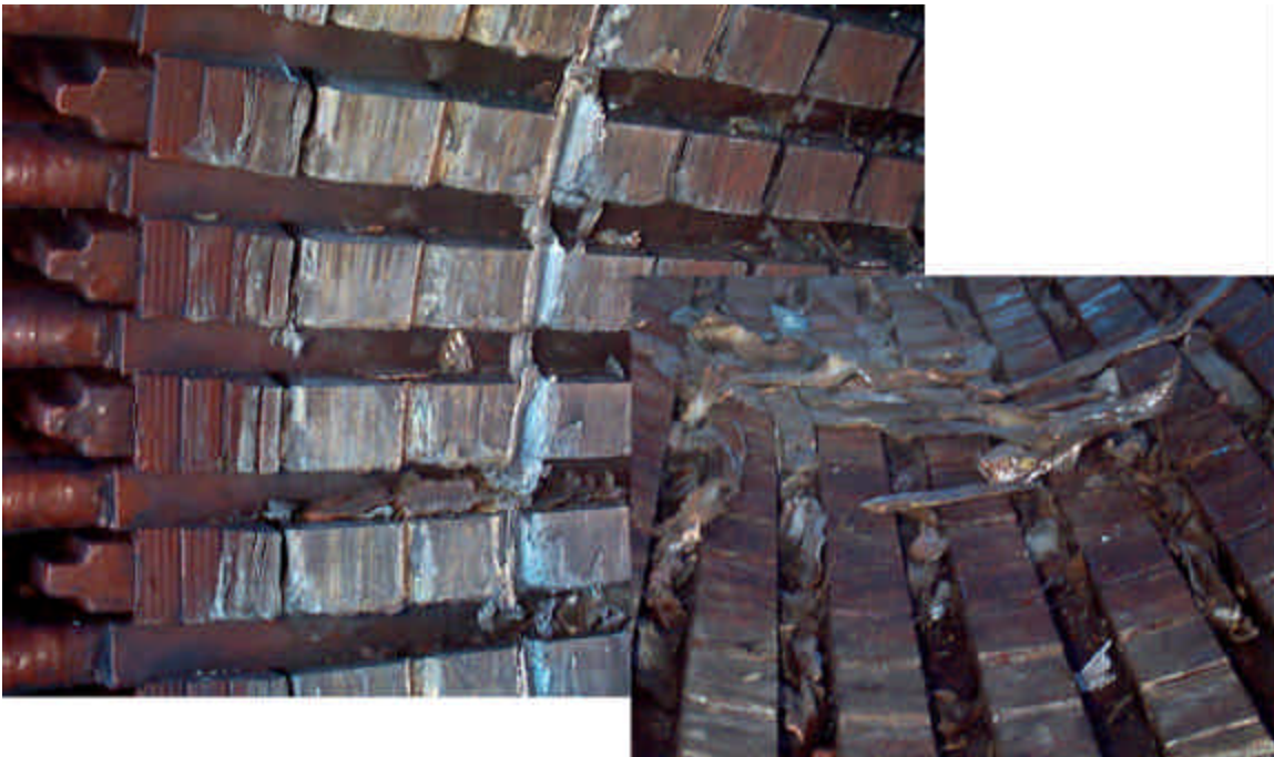
Figure 3: With a rotor wedge displaced at full rotational speed, substantial damage to the stator resulted.
