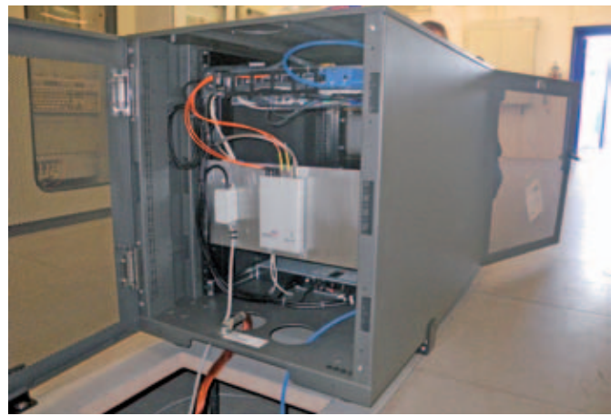
The monitoring server system at the substation in Siems: It captures, logs and provides measured data for the user.
