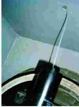
Photo 2. Portion of an Adwel sensor and the Cable Penetrating the Bus Enclosure.
