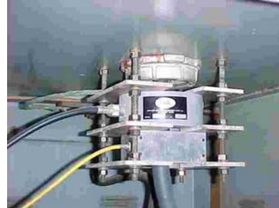
Photo 5. AEP Sensors for Reading EMI. New RFCT Installed Below the Original RFCT.
