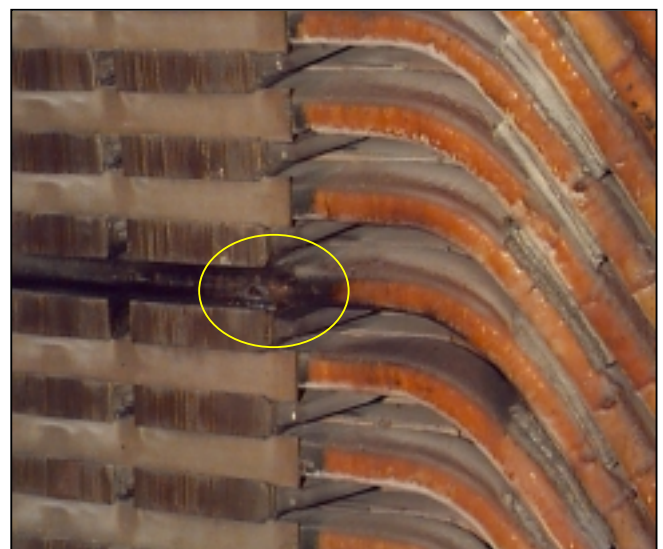
Fig. 8 Insulation failure of motor A.
