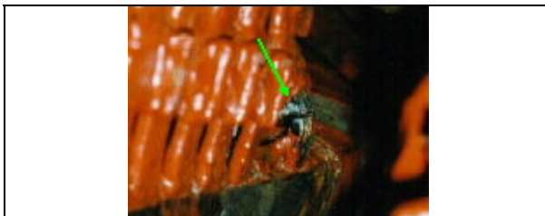
Photo 7. Failure to 1 of 28 parallel circuits in a series connection.
