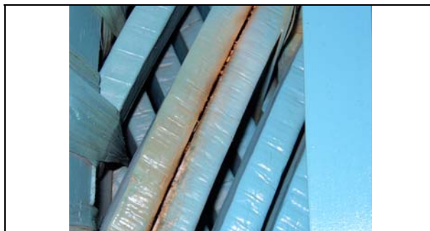
Photo 6. PD at inadequate bar spacing.
