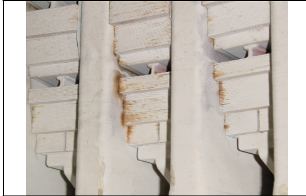
Photo 4. End-of-slot indications of vibration sparking.
