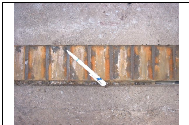
Photo 5. Stator bar failure due to slot vibration sparking.
