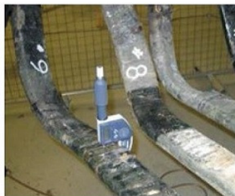
18. Small coil-wound generators made with inappropriate asphalt material post-1970 reintroduced the failure mechanism illustrated in Fig 17. In photo, the remaining groundwall measured 20% of original thickness
