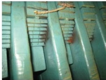
14. Side forces on the top bar likely caused the vibration that led to dusting
