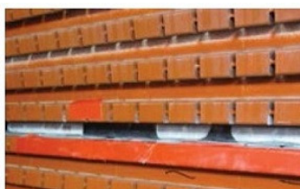
19. Slot partial-discharge activity is in evidence on this modern air-cooled generator
