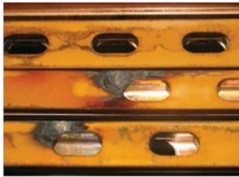
20. Strand shorts in a direct-cooled field are caused by contaminants entrained in cooling air
