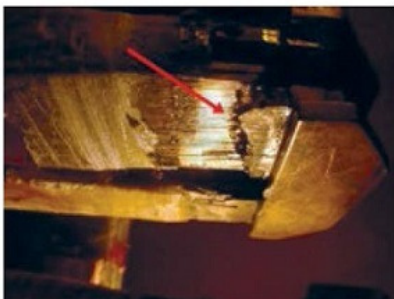
1. Broken bar was caused by absence of series blocking on an endwinding
