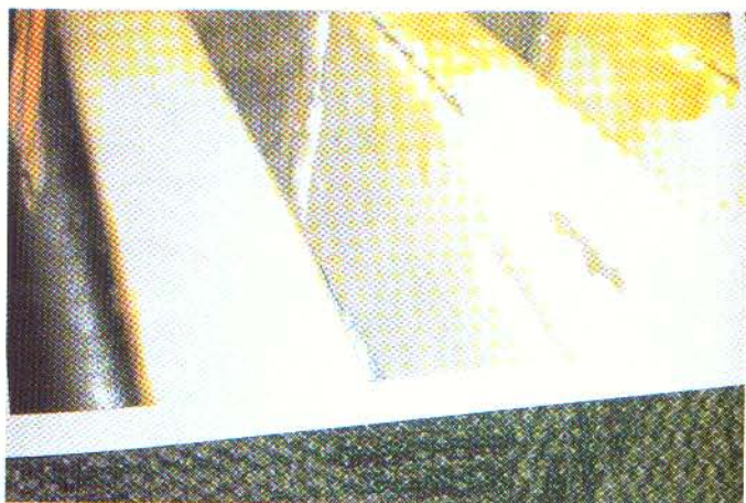
Fig. 7 White powder from PD activity in a small air space in the endwinding between two bars operating at very different voltages.
