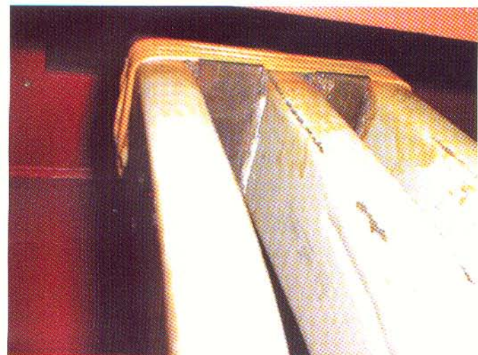
Fig. 5 Small air space between blocking at two phase leads has created PD (white band).
