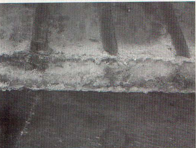
Fig. 3 Example of bar removed from a global VPI stator that failed due to slot discharges. The photo shows the edge of the bar where abrasion and PD damaged the insulation.
