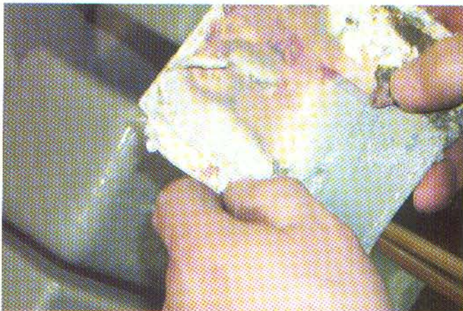
Fig. 6 Nomex used to fill space between phases in different phases. PD activity has eaten into the insulation.
