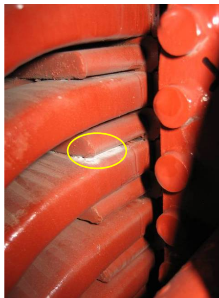
Fig. 10: PD occurring between a core pressure finger and a high voltage coil.
