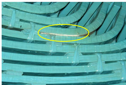
Fig. 8 PD occurring between high voltage coils in two different phases.
