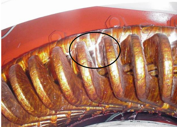
Fig 11: White powder due to fretting at interfaces caused by endwinding vibration.
