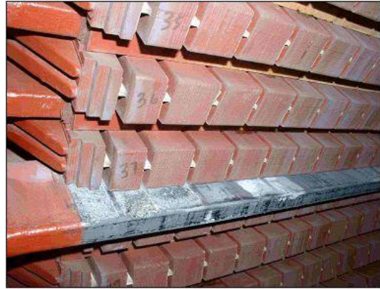
Fig. 5: Bar abrasion due to loose windings in the slot of a turbo generator.
