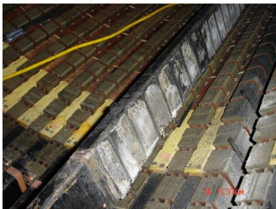
Fig. 7: A neutral end stator bar damaged by vibration sparking.
