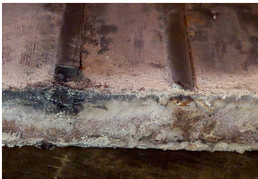
Fig. 6: Damaged bar surface due to loose coils in GVPI stator.
