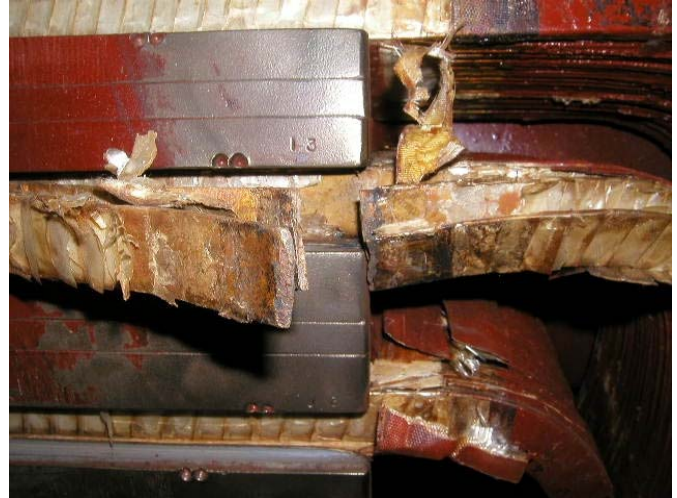
Fig. 10. Two top copper rotor turns with breaks, which have occurred as the coils leave the slot, and the results of the subsequent electrical ground.
