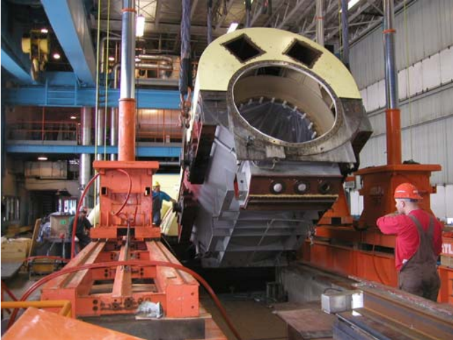
Fig. 14 shows up-righting of generator stator in preparation for a restack of the stator core laminations.
