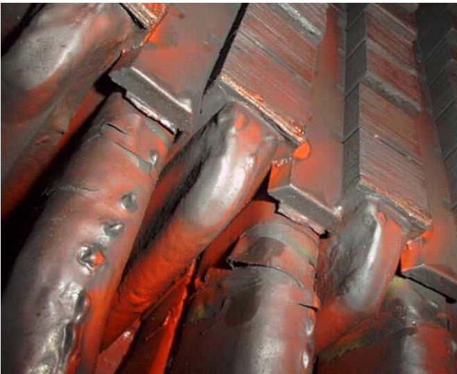
Fig. 2. Evidence of coil girth cracking, often called tape separation, on a 1950s-vintage generator with asphalt-based insulation.
