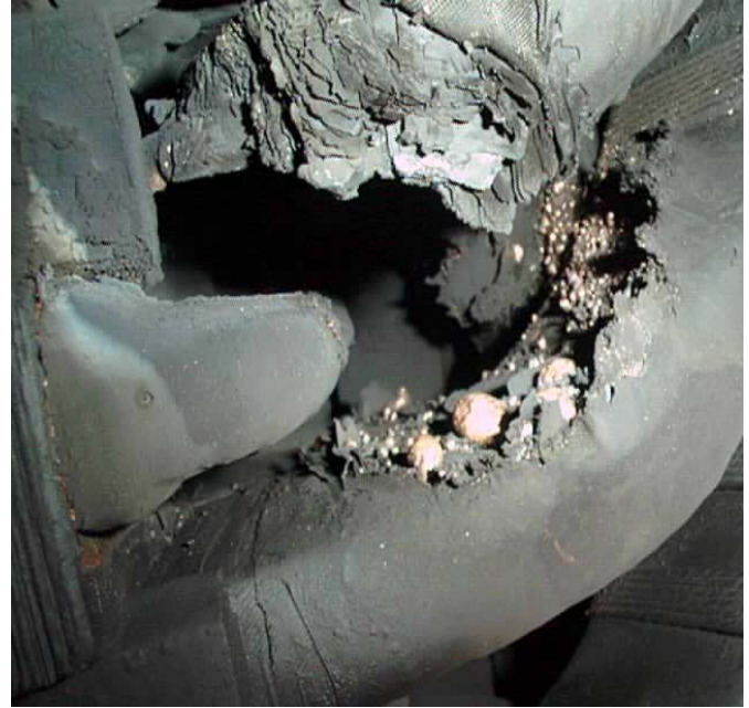
Fig. 3. Girth cracking in this particular machine, lead to a coil electrical ground fault that also damaged the stator core iron.
