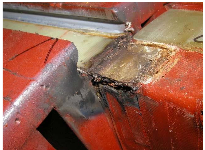
Fig. 13. Rotor top turn cracking caused an electrical ground fault from the rotor turn, through the ground insulation and to the rotor forging.
