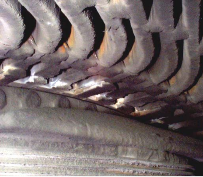
Fig. 1. Extensive partial discharge activity in stator winding, shown by its white "powder-like" appearance, can deteriorate the insulation, eventually causing an electrical ground fault.
