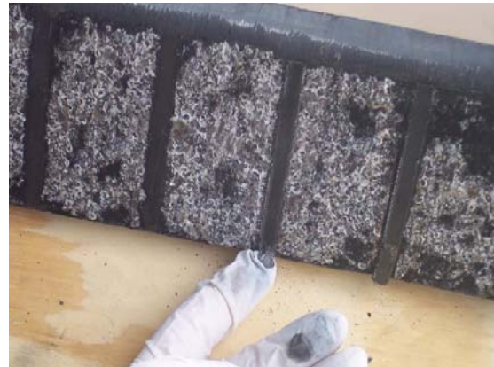
Figure 12. Photo of spark erosion damage on a winding from another OEM. This winding failed after 33,183 hours of service and less than six years of operation v .
