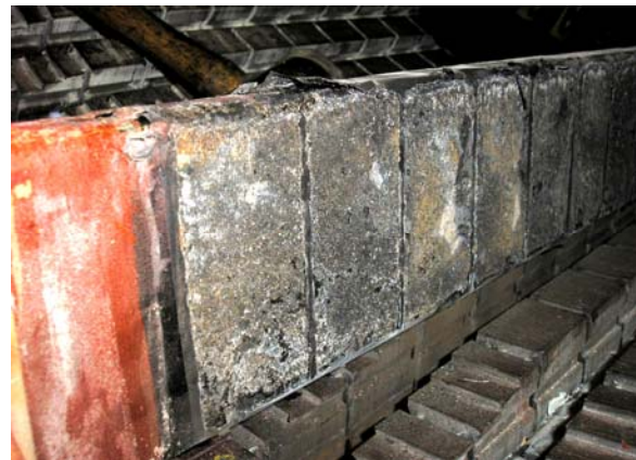
Figure 1. Stator bar with spark erosion damage being removed from slot.
