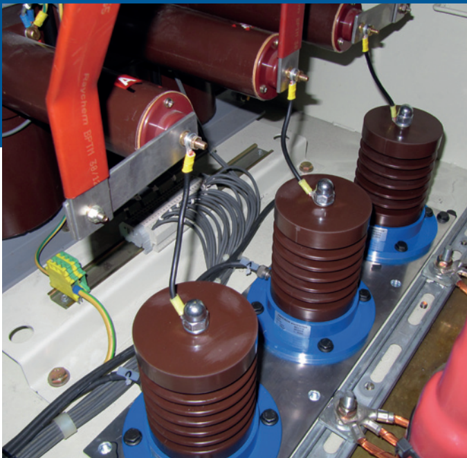
Fitted directly to the generator's bus bars: Capacitive couplers for detecting partial discharge signals.
