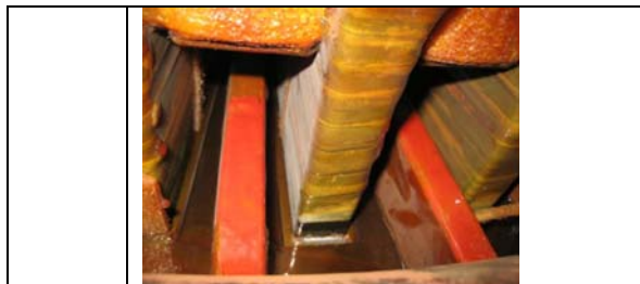
Photo 16. Stator bar surface conditions misdiagnosed as partial discharge.
