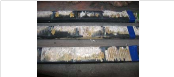
Photo 6. Slot discharge primarily due to poor slot conductive coatings.
