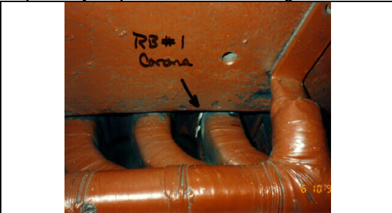
Photo 17. Arcing damage at end-grading junction.
