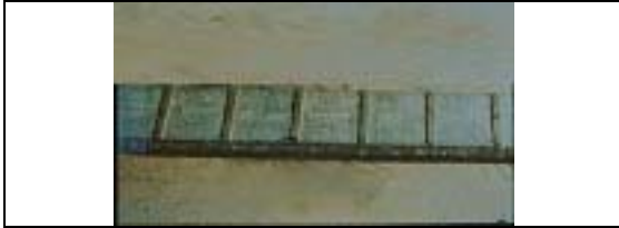
Photo 5. Bar that has been abraded due to looseness in the slot.
