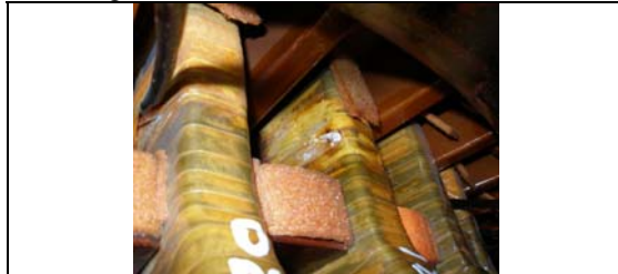
Photo 15. Stator bar surface conditions misdiagnosed as partial discharge.
