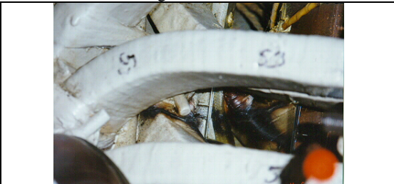
Photo 19. Endwinding arc damage during shipping hipot.
