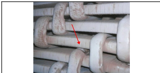
Photo 10. PD on a bar tie at a line-to-line phase break.
