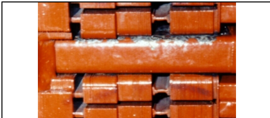
Photo 8. Major slot PD due to inadequate slot grounding paint system.
