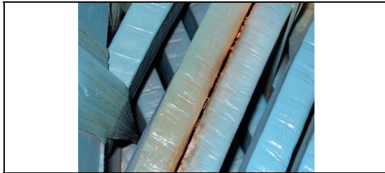
Photo 9. PD at a line-to-line phase break.
