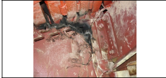
Photo 20. Arc resulting from water dripping onto endwinding. Outdoor unit.
